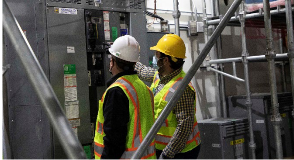
Electrical system testing in the Mechanical Electrical Building supporting the UPF.
